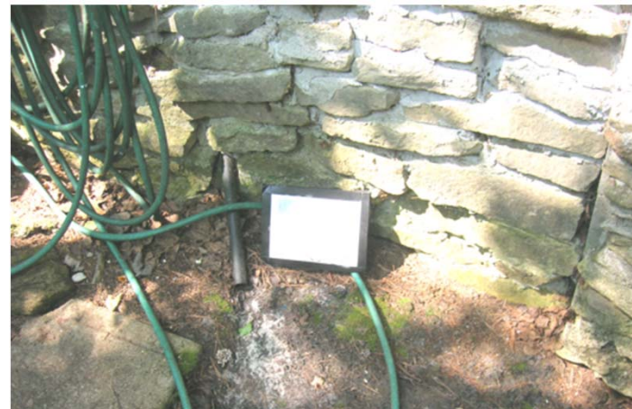
Greywater Discharged to Surface
