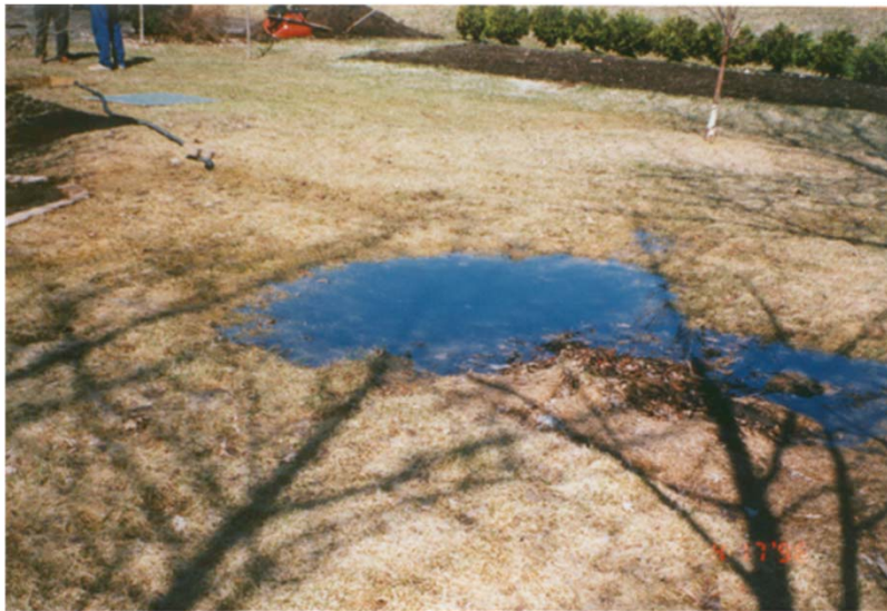
Effluent Pooling Over Bed
